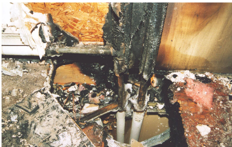
(a) Ignition of wood floor/ceiling assembly from a hot-water supply pipe (left pipe in the photo) (Courtesy Ken Swan)
